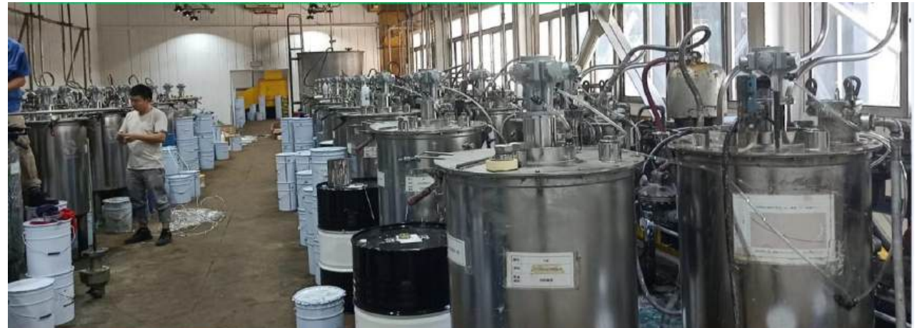
Qingling Motors 250L Air mixers update project
